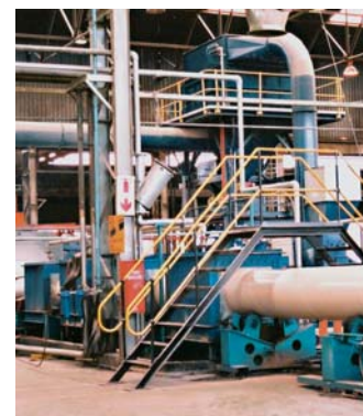
FBE coating line
